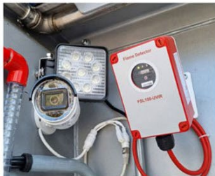
Flame and Smoke Detection System
